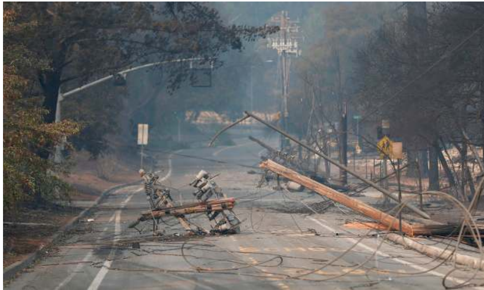
3 4 5 6 7 8 9 10 11 12 Broken and Burned Electrical Equipment in Santa Rosa, California 8
