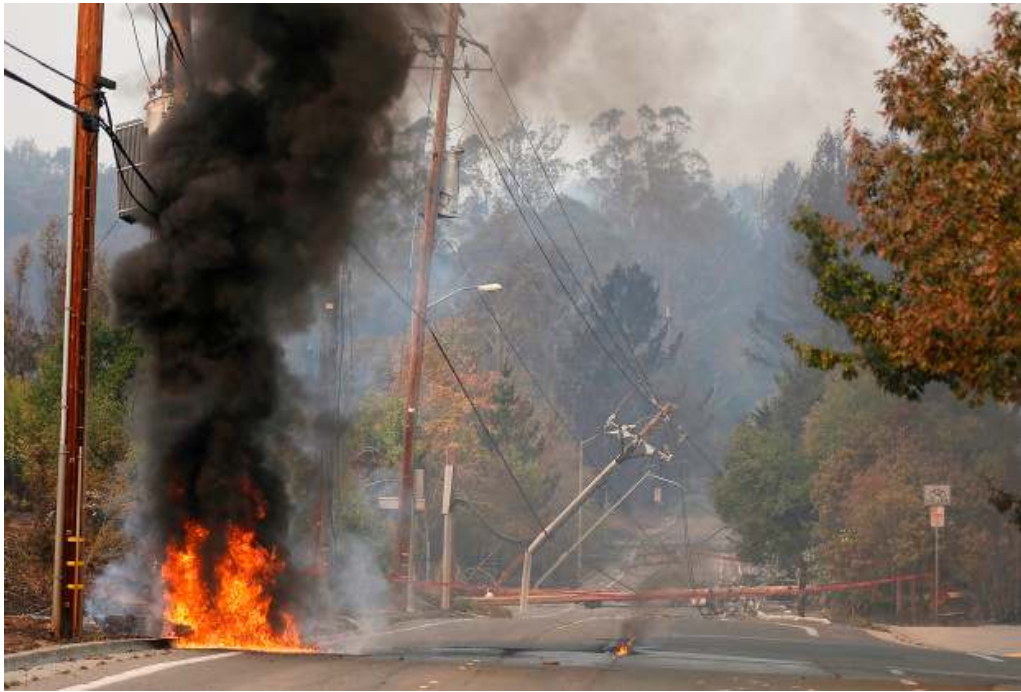
3 4 5 6 7 8 9 10 11 12 13 14 Failing PG&E Equipment Along Parker Hill Road in the Tubbs Fire 4
